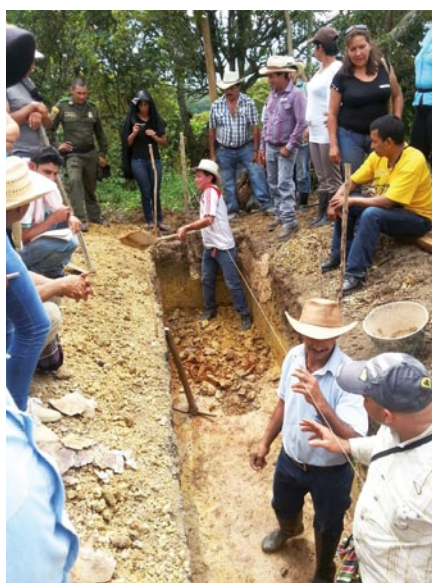
Site preparation for the installation of a tubular biodigester during the field workshop in Guadalupe, Santander
