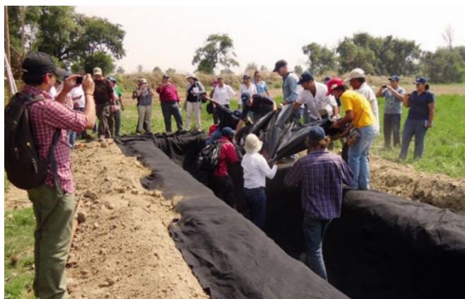
Installation of a tubular biodigester during the annual RedBioLAC conference in Mexico
