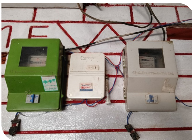
Figure 6: Energy meters of two MHP plants with a converter in the middle
