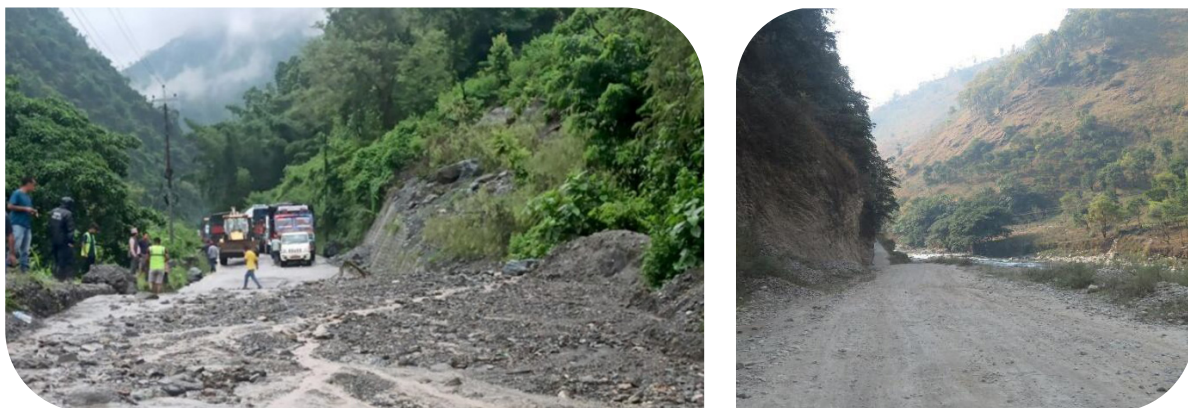
Figure 4: Damaged road in Galkot-Badigad-Nisikhola Corridor
